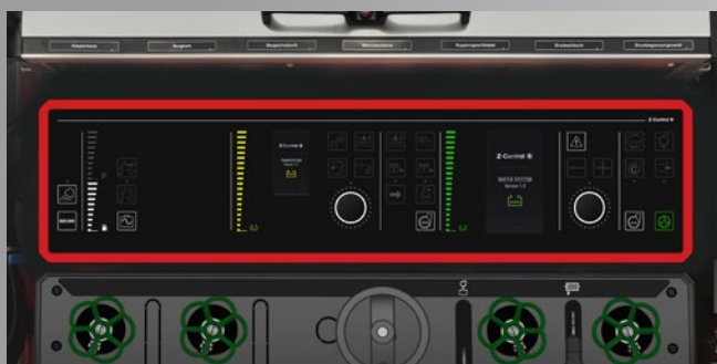
Control and Operation
